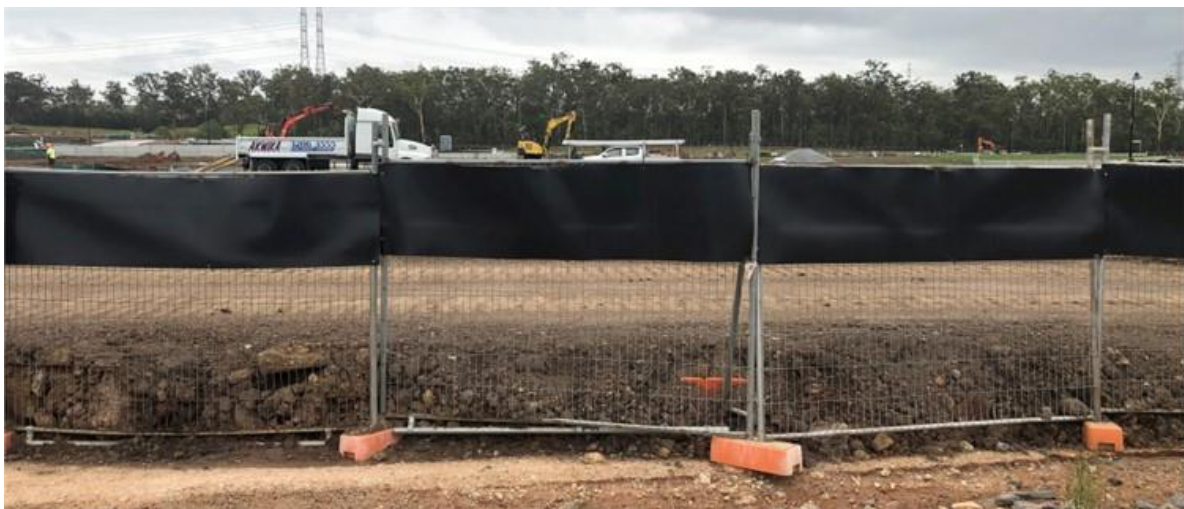
Inset 1: Indicative temporary fauna exclusion fencing aligning a construction site.
