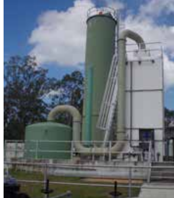
TREATMENT: The plant’s bio-trickling filter and new activated carbon unit.
