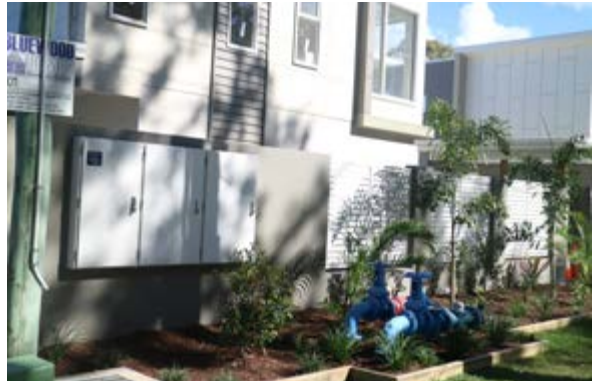
The service boxes visually blend with the colour palette and the landscaping will mature to soften the appearance of the services.
