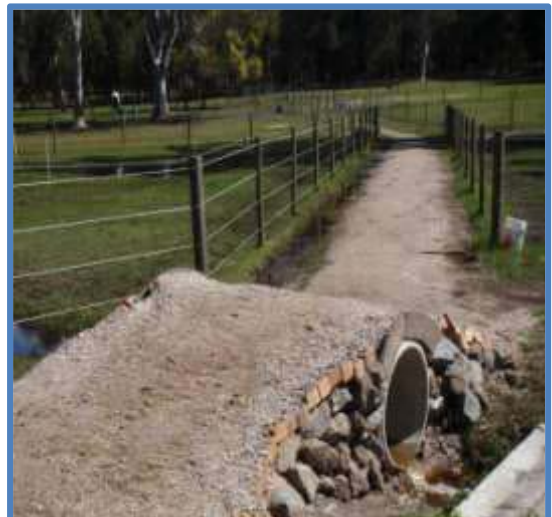
After: Formal causeway to prevent leeching of nutrients and sediment into the creek.
